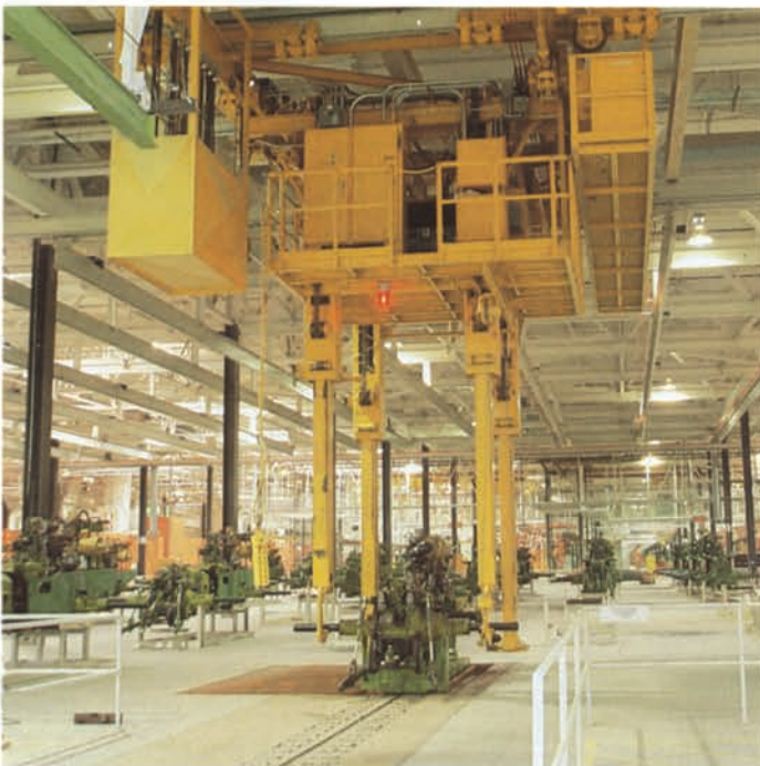
Chassis storage using horizontal automatic storage/retrieval system with two bridge cranes and chassis carriers.
